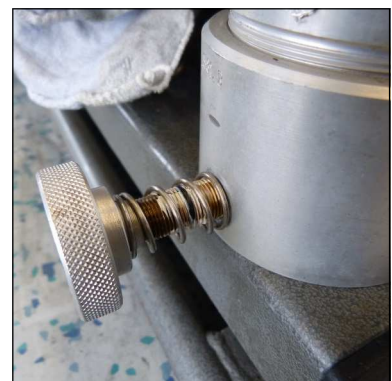
Abb. 6 - O-ring, condensate drain valve
