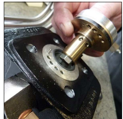
Fig. 4 - Ensure correct valve position (centre pin)
