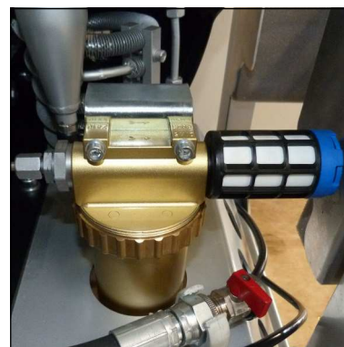
Oil / water separators final stage
