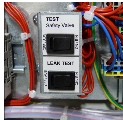
Leak test switch (lower)
