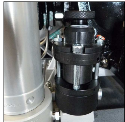
Fig. 2 - Safety valve 3rd stage
